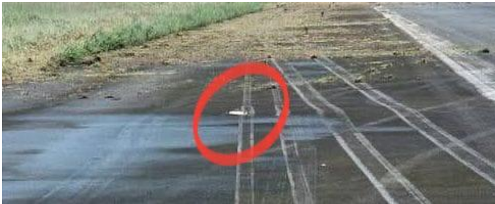
Figure 3. Damaged runway edge light L13
