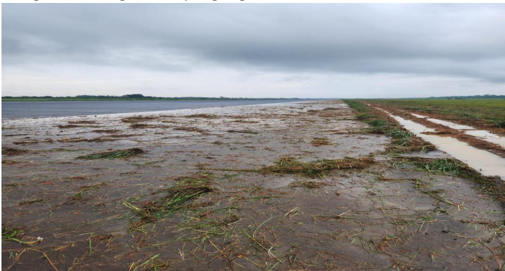
Figure 4. Tire rut along the runway
